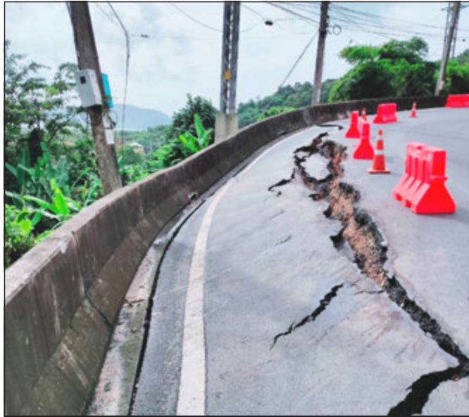
Heavy rains washed away the earth supporting the outer lane, leading to the outer part of the lane to collapse. Photo: Phathada Sae-Lim / Facebook
